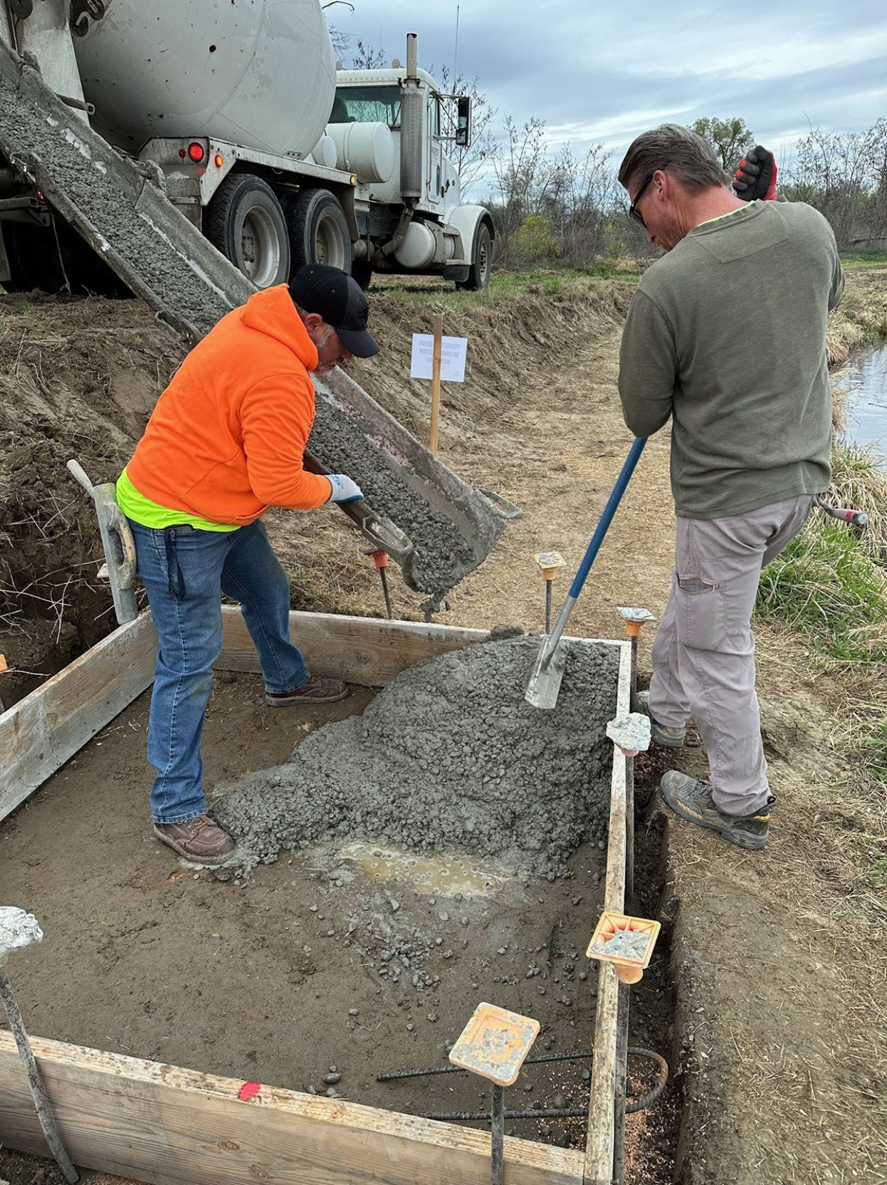
Volunteers from OPCMIA Local 72 poured pads prior to the fishing dock installation.
